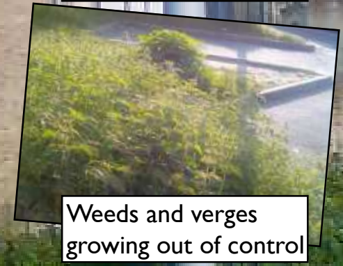
Broken kerbs a risk to cars and pedestrians
