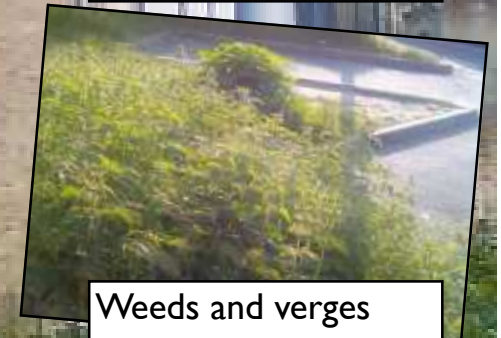
Broken kerbs a risk to cars and pedestrians
